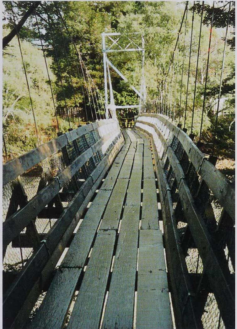
The Major Jones Bridge was hit by a pine tree being washed down the river. Note the kink, caused by the weight of the debris on the broken sway wires
