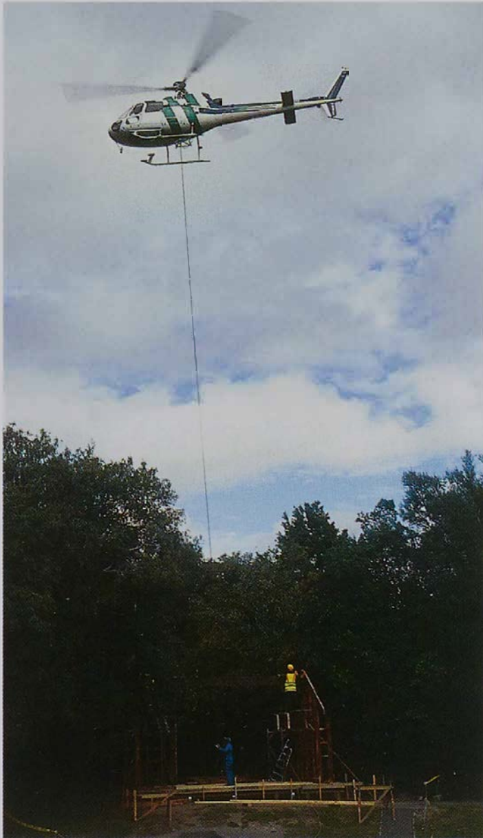
Peter Masters of Taupo Helicopter Services lifts the main structural beam for the new kiosk into place
