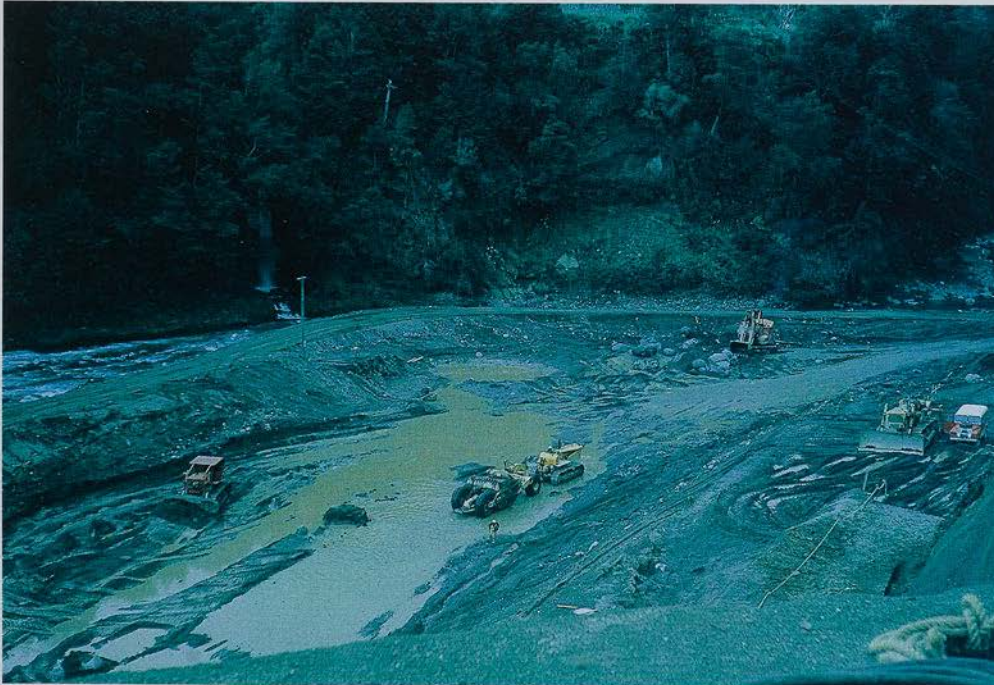
Construction of the coffer dam to divert the Tongariro River while the Poutu Intake is built - April 1969
