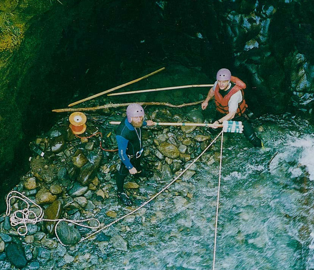
Tom May (left) and Glenn Maclean prepare to lay the charge. Photo Rob Hood
