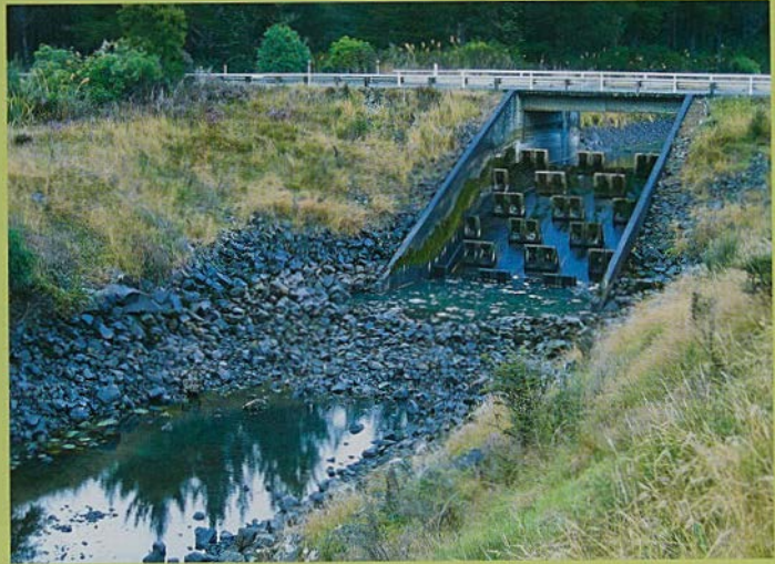
The fish collect at the base of each drop structure. Photo by: Mark Venman
