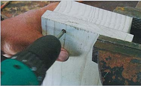
Ensure the screws are posidrivn or countersunk below the timber surface Photo by: John Webb
