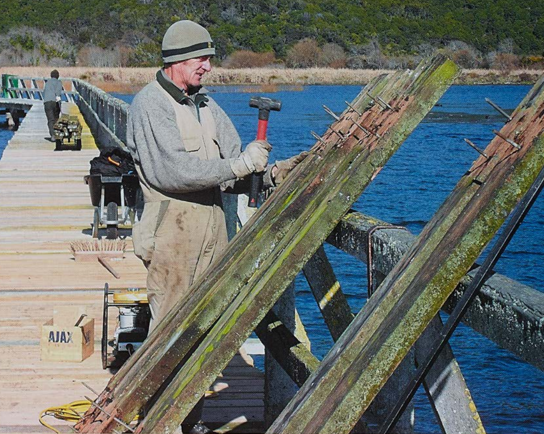
Visitor Assets Ranger Paul Prendergast replaces the timber decking during the restoration of the Tokaanu Wharf
