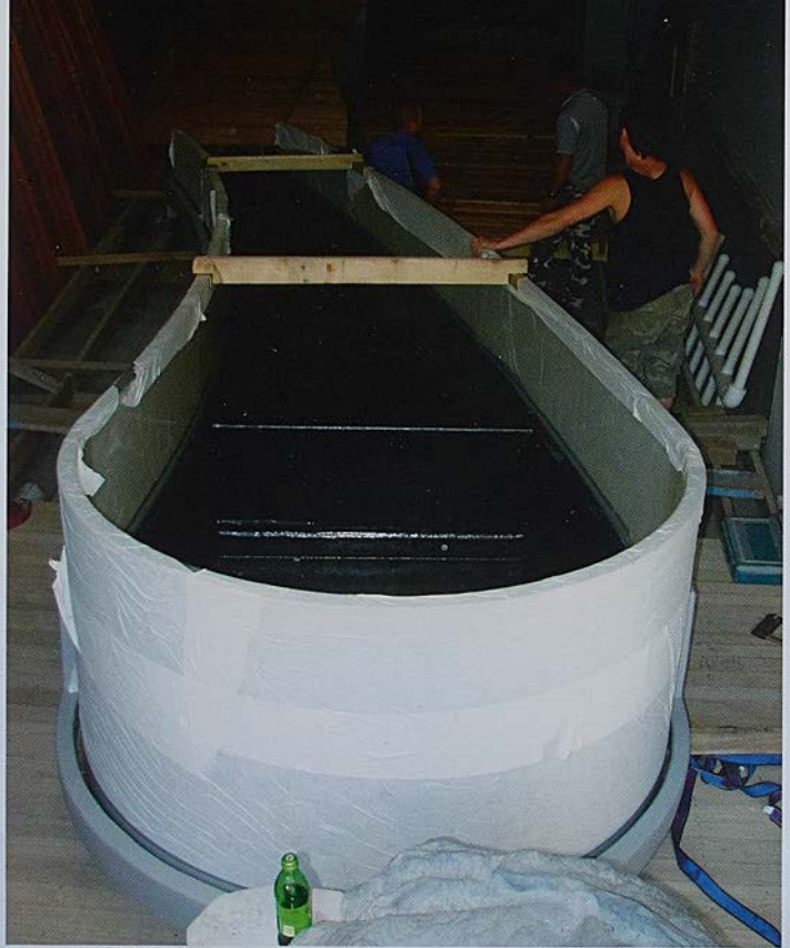
The first half of the centerpiece transition or "riffle" tank arrives Photo by: Randal Hart
