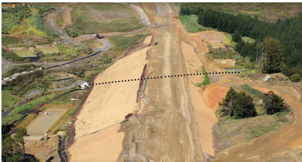
Figure 3-32 At left, a major headwater reach (5.4 km 2 source zone upstream) of the Mahurangi is one of two tributaries that have been buried under the Puhoi-Warkworth Expressway. Instead of a bridge (viaduct) that would retain many of the natural features and much of waterway connectivity, this system comprises three 130 m long culverts. Barriers such as culverts strongly inhibit lateral and longitudinal connectivity, and any potential for local river evolution.
