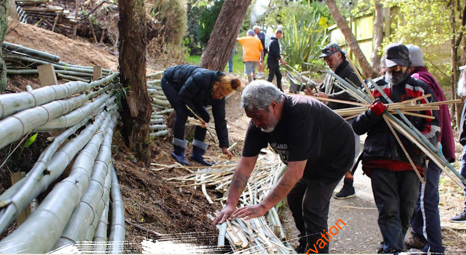
Excellent progress in removing bamboo and reusing it for terrace wall by the Street Guardians Group. Photo: Tomorrow Inc
