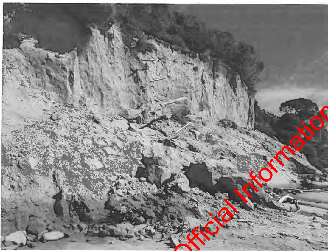
Image 4 Example of hanging fence line that has been subject to the eroding cliff line
