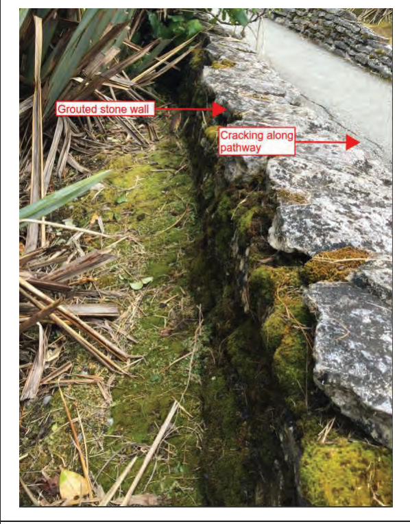
Photograph 4: Grouted stone wall downslope of crack.
