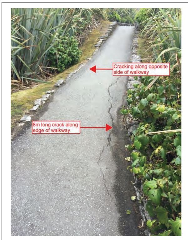
Photograph 1: Location 7 crack location.
