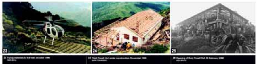
23 Flying materials to hut site, October 1999 24 Good Powell Hut under construction, November 1999 25 Opening of Wood Powell Hut, 26 February 2000
