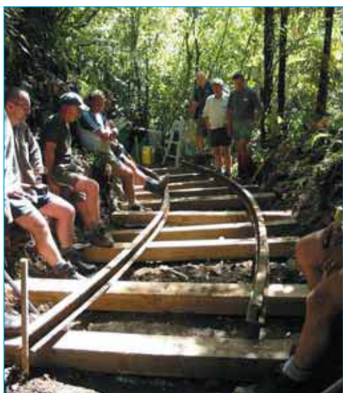
Tangible history. Recreating a past tramway at Sheridan Creek, Otaki Forks, Tararua Ranges. Photo: P.J. Mahoney
