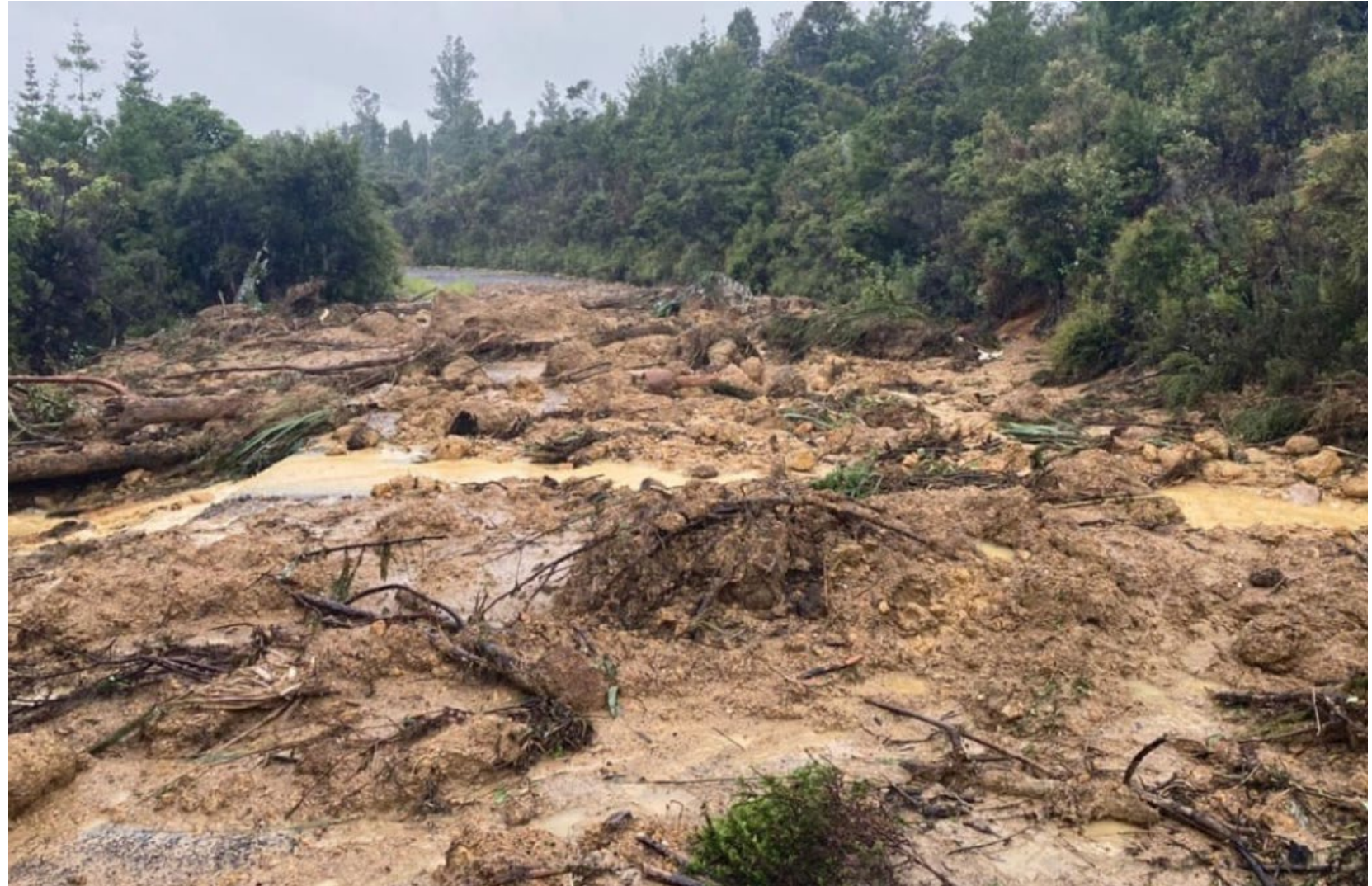
Photo: A slip covering the road at Sailor's Grave, near Tairua. Source: Supplied to NZ Herald/ Leonard Powell
