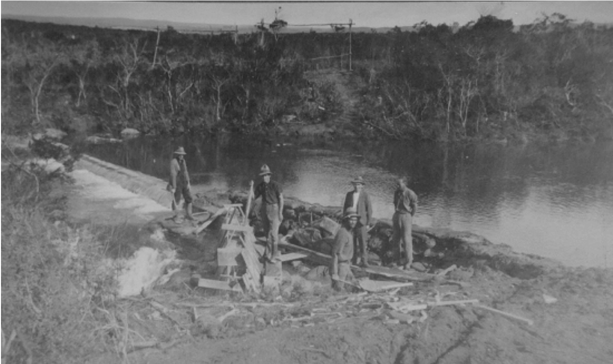
Figure 2: Construction of the concrete dam and diversion weir at Rainbow falls (BOIEPB).
