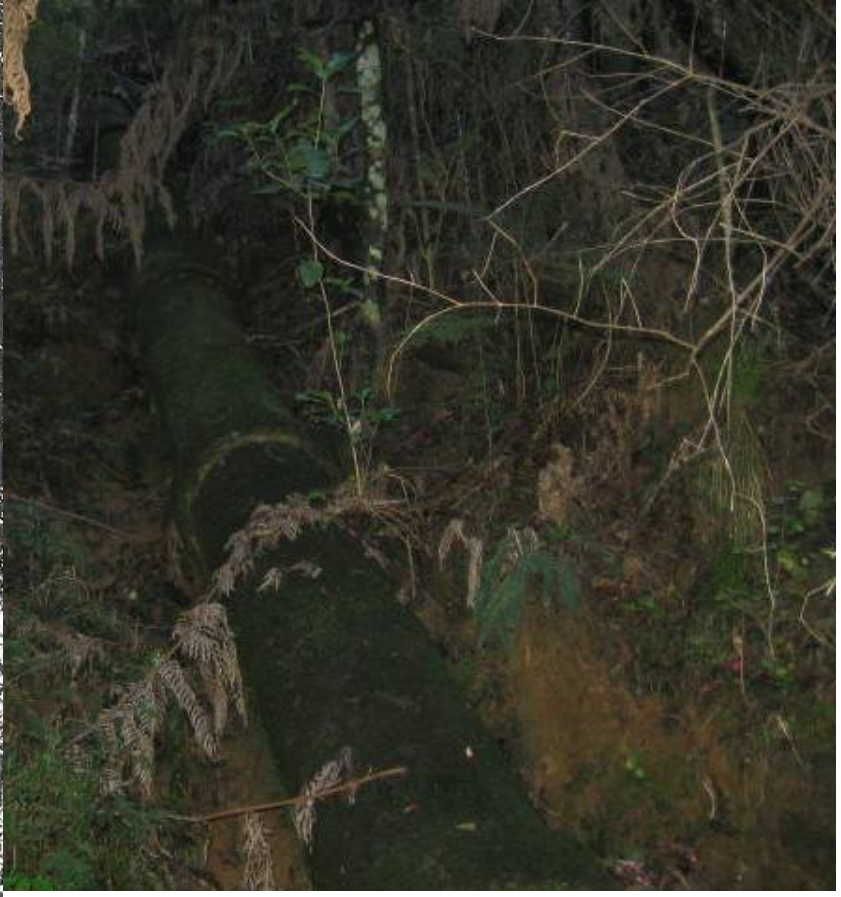
Figure 13: Part of the concrete pipes today still intact but not highly visible under vegetation (DoC 2011)
