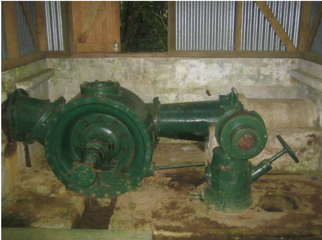
Figure 15: The Francis turbine and generator in the reconstructed powerhouse (DoC 2011)
