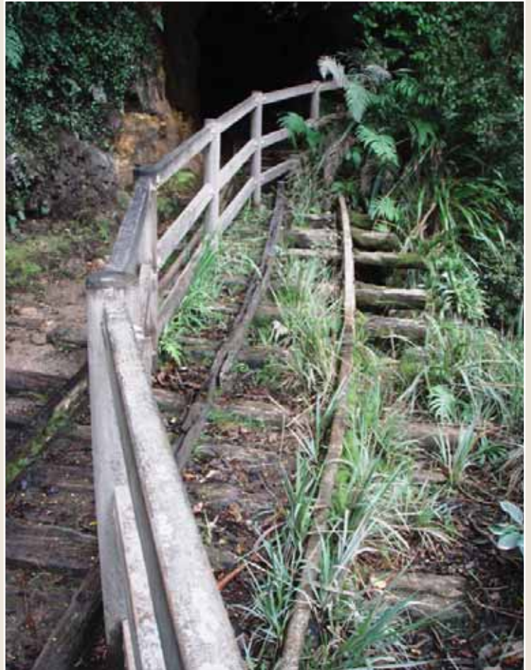
Photo 72: Slipped section at the south western end of the Mangatini tunnel.
