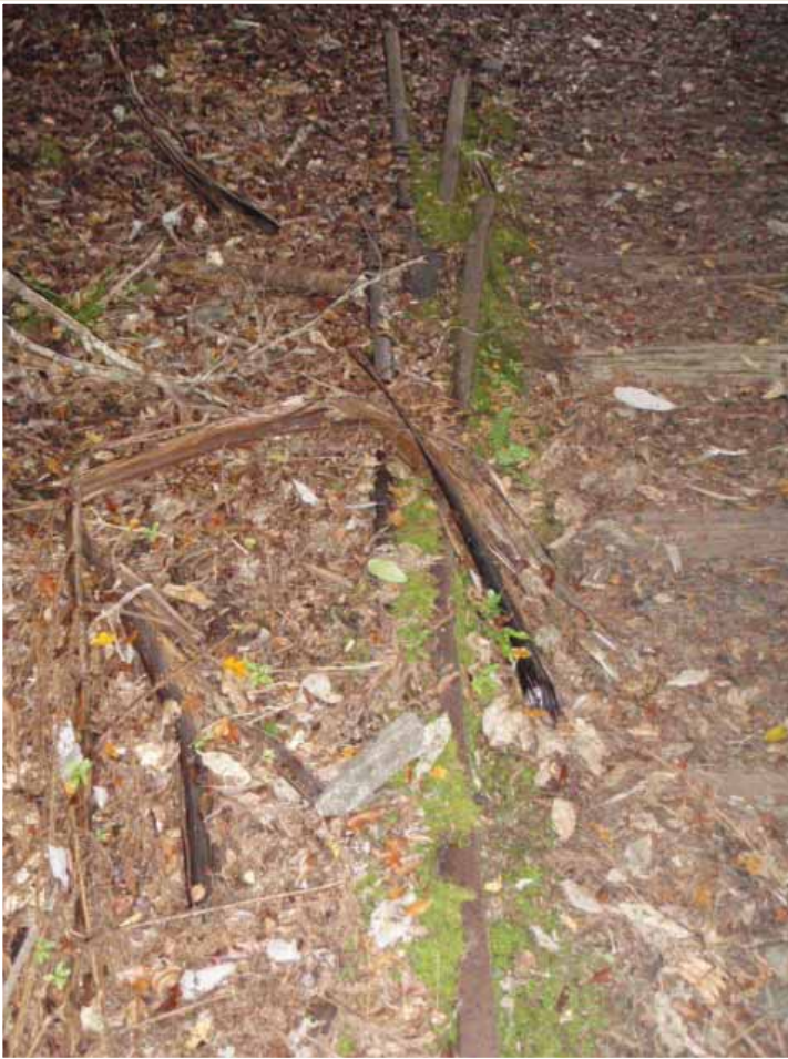
Photo 83: A 'frog' at a set of points where rails for the coal and timber trams split to provide sidings access. N. COOKE 2008
