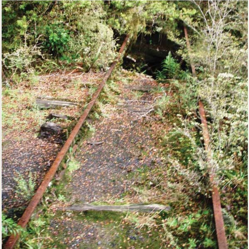
Photo 59: Left - Bridge site near Watson's Mill Shelter. The rails hang in mid air as the bridge has been washed away.
