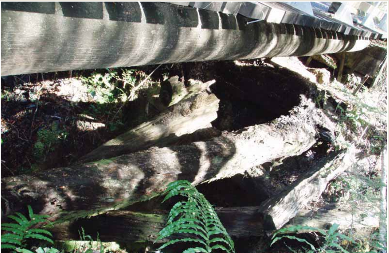
Photo 46: Modern bridge constructed over old bridge with old beams still left in-situ.
