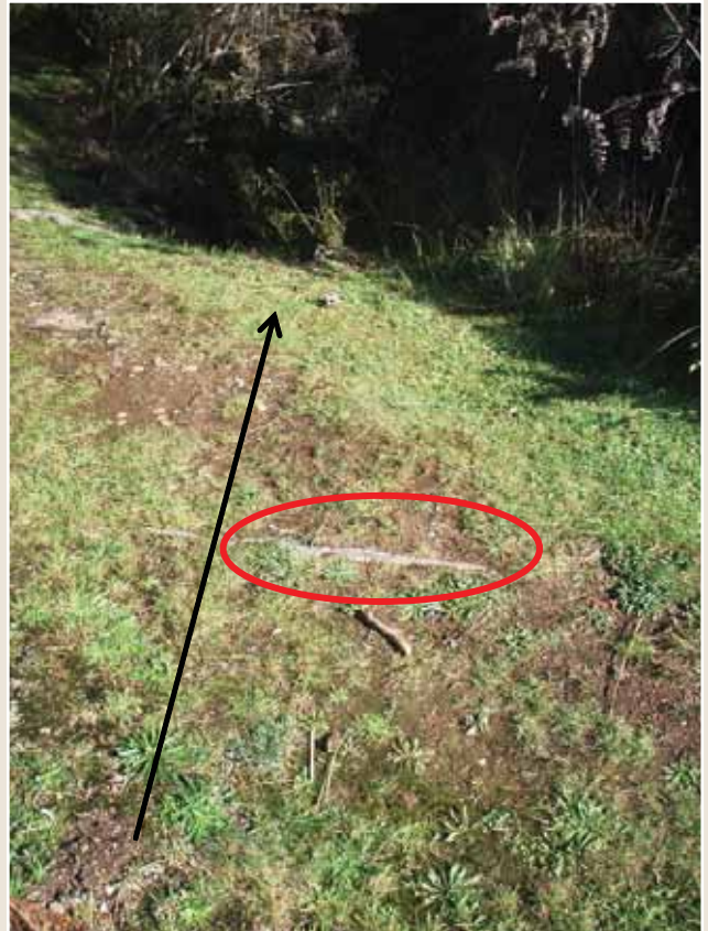
Photo 26: Tramway alignment from mine entrance, where the high level siding intersects with the walkway. The line of the tram is marked by an arrow. A sleeper exposed in the track surface has been circled.
