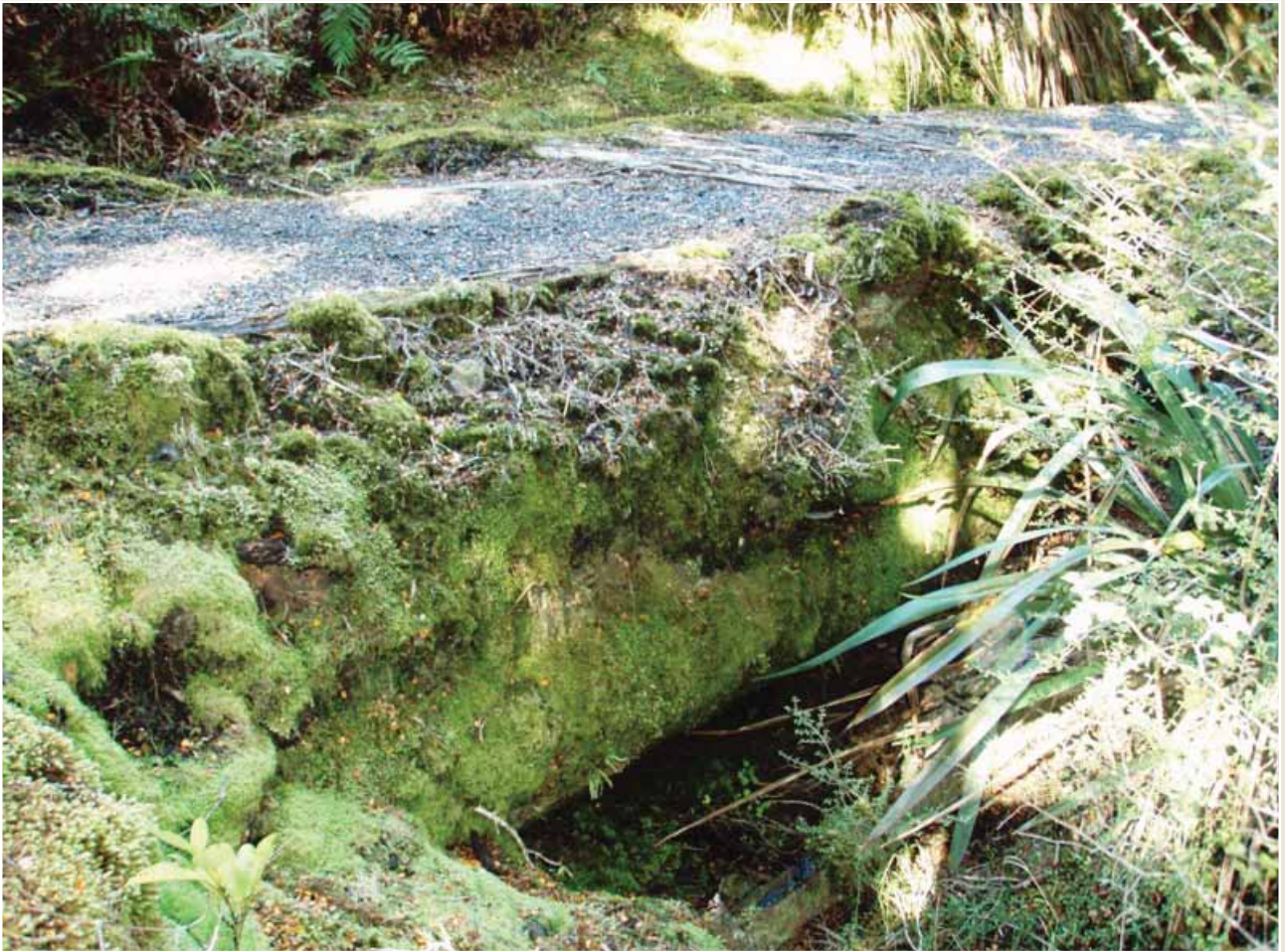
Photo 45: Original bridge. The bearer is marked with a dashed line. Tram surface with sleepers can be seen on top.
