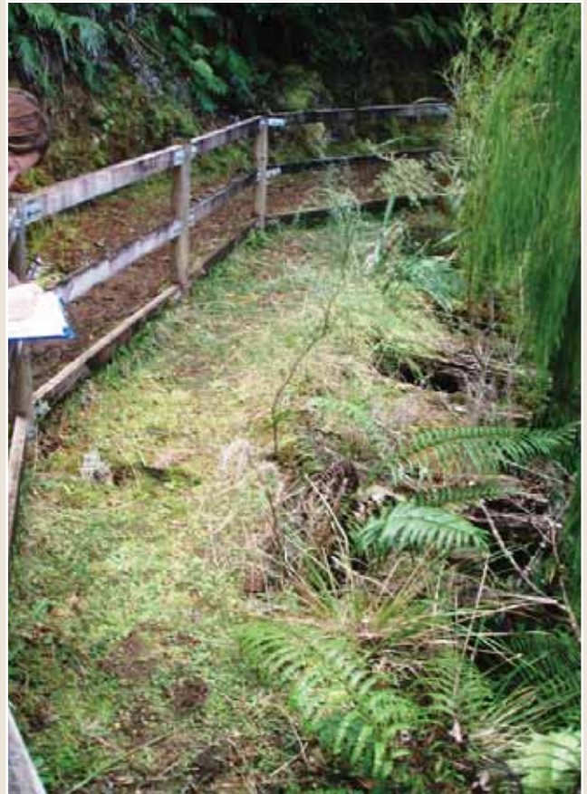
Photo 56: Section of tramway being undermined.
