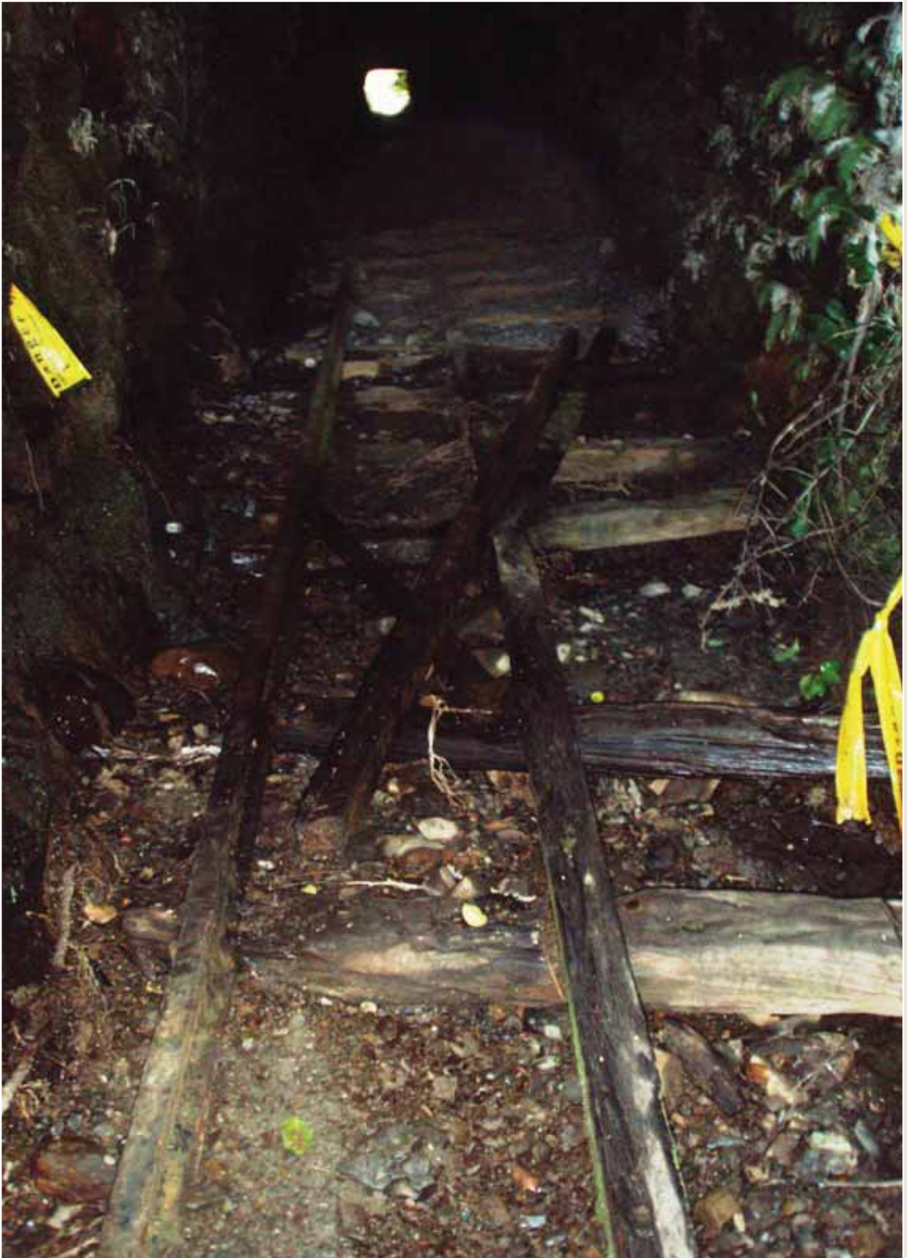
Photo 22: Centre brake rail, sleepers and rail, looking into Papa Tunnel from its west entrance. The eastern entrance can be seen in the distance.
