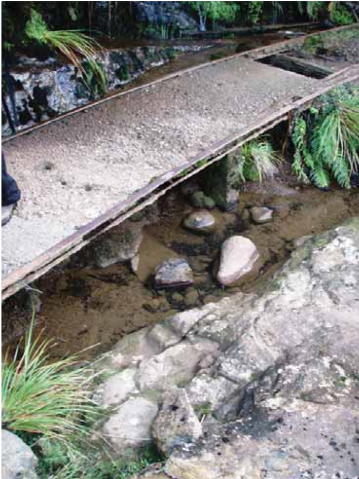
Photo 71: Waterfall undermining rail formation under concrete slab.
