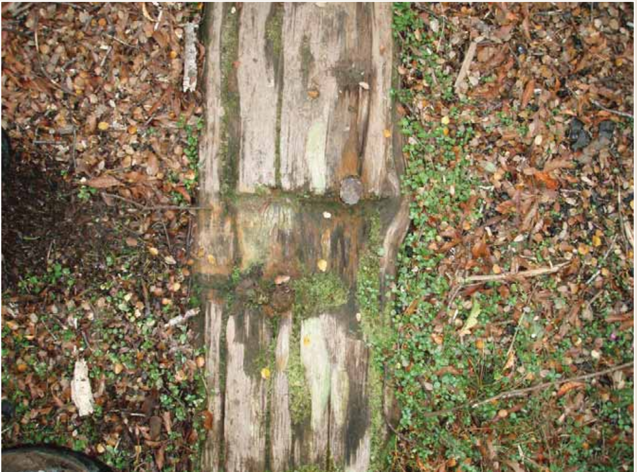
Photo 55: Sleeper with a rail notch adzed into it.
