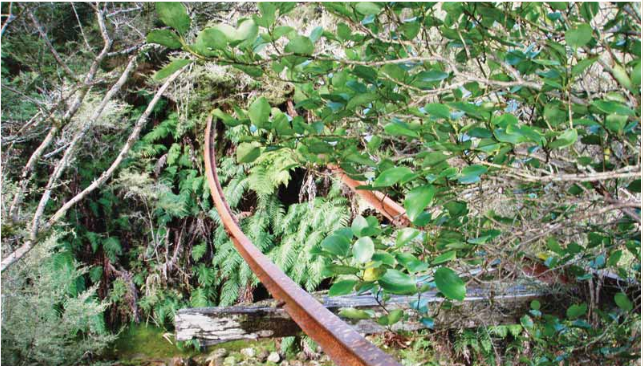
Photo 60: At the other end of the bridge only the rail and a few precarious sleepers remain.
