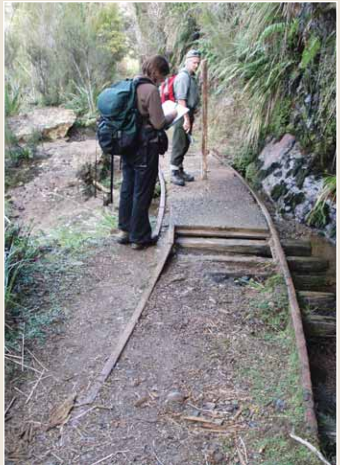
Photo 62: A section of the concrete slab bridge which has been undermined by water.
