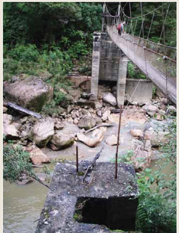
Photos 69 and 70: The Ngakawau Suspension Bridge looking to the true right, and detail of abutments and cables in the river bed below the bridge.
