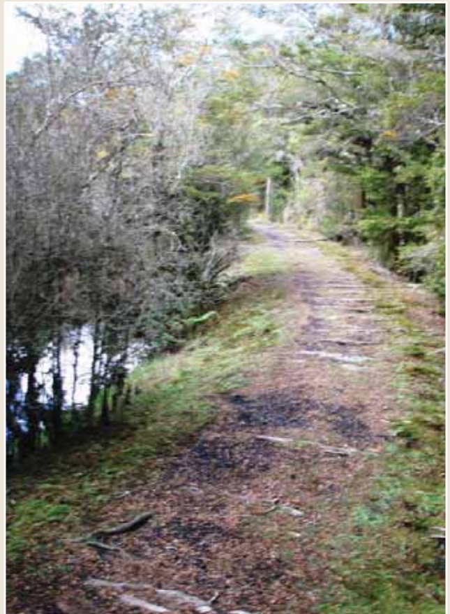
Photo 53: Embankment formation with sleepers exposed
