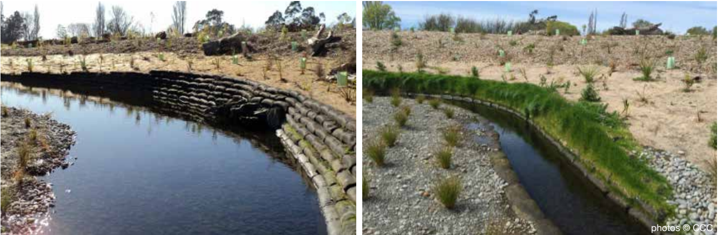
FIGURE 7: Steep banks stabilised with geotextile bags along a new alignment of Kaputone/Kā Pūtahi Creek. Bags in the left image have grass seed sown within the bags, whereas bags on the right were hydro-seeded, resulting in a faster strike rate. The same mix of native grass seeds were used.
