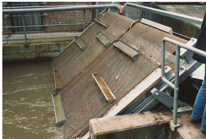
Figure 5.64: Travelling screen with transportation troughs at the hydropower plant Hadamar in the Elbbach (Hessen, Germany): The troughs with fish being transported therein will be emptied into an irrigated bypass that leads to the tailwater. The installation consists of a 40 mm-screen with screen cleaning machine connected in front. The travelling screen works intermittently.
