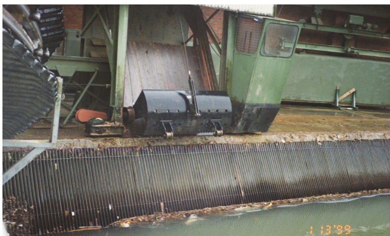
Figure 5.32: Screen with rope driven screen cleaning machine at the power plant Ahl on the Lahn river (Rhineland Palatinate, Germany)
