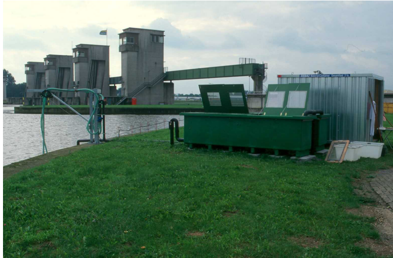
Figure 5.118: MIGROMAT® on the bank of the Maas river in Alphen (The Netherlands)
