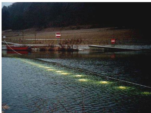
Figure 5.56: Chain of lights in operation at the hydropower plant Dietfurt an der Altmuehl (Bavaria, Germany)
