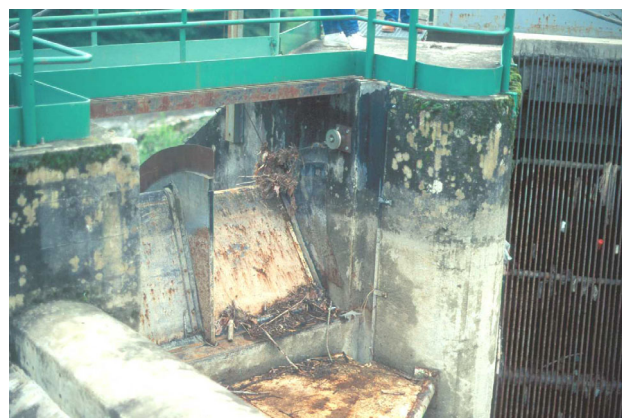
Figure 5.72: The sluice of the hydropower plant Soeix on the Gave d'Aspe river (France) directly above the screen has been successfully converted into a bypass for salmon smolts (view of drained head-water channel)
