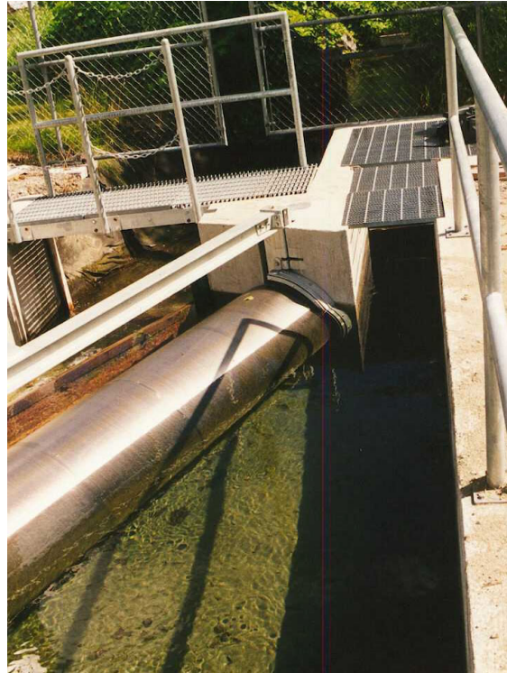
Figure 5.85: Fish protection facility at a water intake employed for irrigation purposes in a tributary of the Yakima river (Washington, USA): drum screen made of perforated panels ( d = 3.0 mm) with a diameter of 0.8 m arranged inclined to the flow direction; the bypass inlet is arranged at a pointed angle
