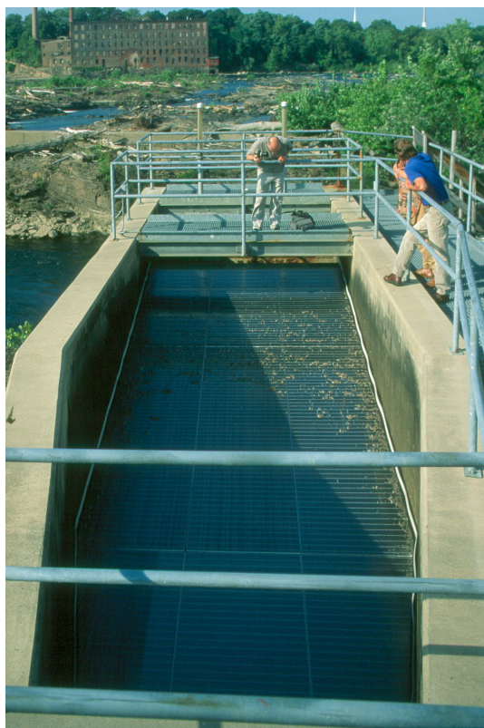
Figure 6.10: Very flat inclined Wedge-Wire-Screen at the bypass outlet at the Holyoke-Dam on the Connecticut river (Massachusetts, USA)
