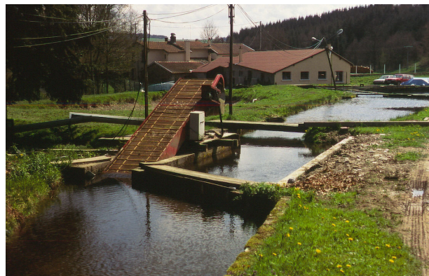
Figure 5.43: Travelling screen at a water intake structure of the fish hatchery d'Augerolles (France). It serves for the removal of flotsam from the inflowing water
