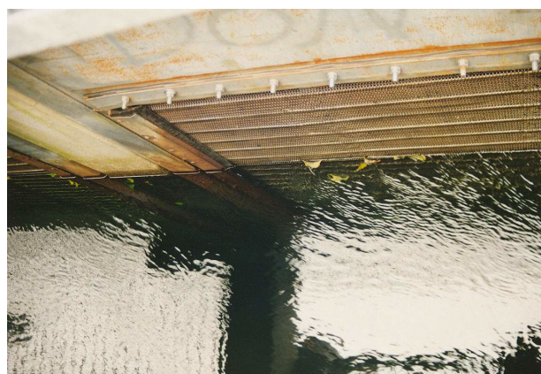
Figure 5.45: Vertically travelling screen of stainless steel fabric with a clear width of 3 mm at the hydropower plant Winooski (USA, Washington State). Flotsam and fish will be transported by the tangential component of the approach velocity. The screen is sealed against the structure with rubber lips at the bottom and the sides.
