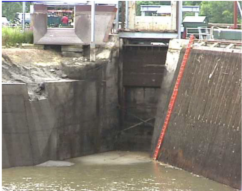
Figure 5.101: Detail of figure 5.100: Screen and flushing gate. The gate was immersed and illuminated in order to create a surface-near bypass opening (HARO, 2000)
