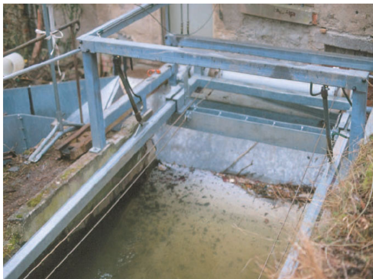
Figure 5.109: A Wedge-Wire-Screen installed at an angle of \alpha = 24^\circ with a clear width of d = 5 \text{ mm} and a traversing bypass channel at the Floecks-muehle (mill) in the Nette river (Rhineland Palatinate, Germany)
