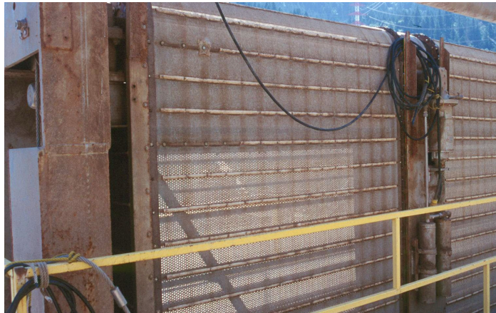
Figure 5.95: Bonneville power plant (Columbia river, Washington State, USA): Travelling screen made of plastic. The picture shows the entire unit which is pulled from a shaft in the feeding channel to the power house
