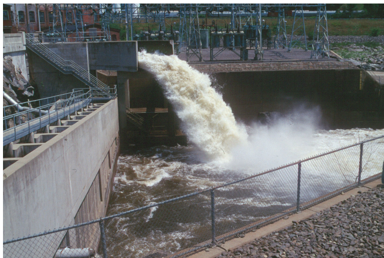
Figure 5.69: The inflow of the bypass at the hydropower plant Bellows Falls on the Connecticut river (Connecticut, USA), is situated approximately 9.0 m above the level of the tailwater
