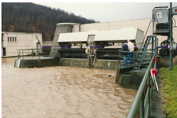
Figure 5.4: Intake of the hydropower plant Wahnhausen on the Fulda river (Hesse, Germany)
