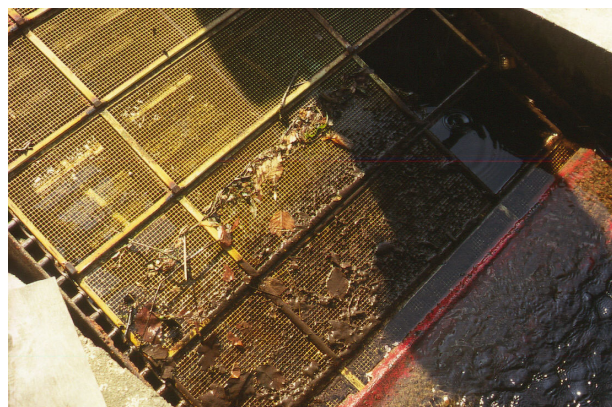
Figure 5.44: Detail of figure 5.43: The screen consists of individual foldable sections of close meshed grids that lean on a supporting construction. Identifiable are driving chain and stiffening material
