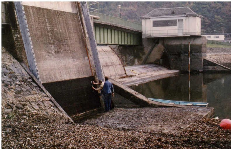
Figure 5.30: Submerged levelscreen in front of the hydropower plant Obermaubach on the Rur river (North Rhine Westphalia, Germany). The upper edge of the screen will be about 2.0 m below water level if the reservoir is filled
