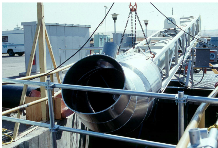
Figure 5.61: Spiral pump of the Tracy Fish Facility at the estuary of the Sacramento-River (California, USA)
