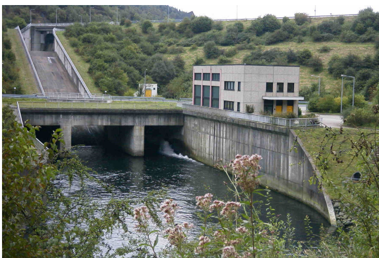
Figure 5.1: Whether downstream fishways are necessary to guarantee a free passage at dams has to be evaluated in individual cases (Wupper Dam, North Rhine Westphalia)
