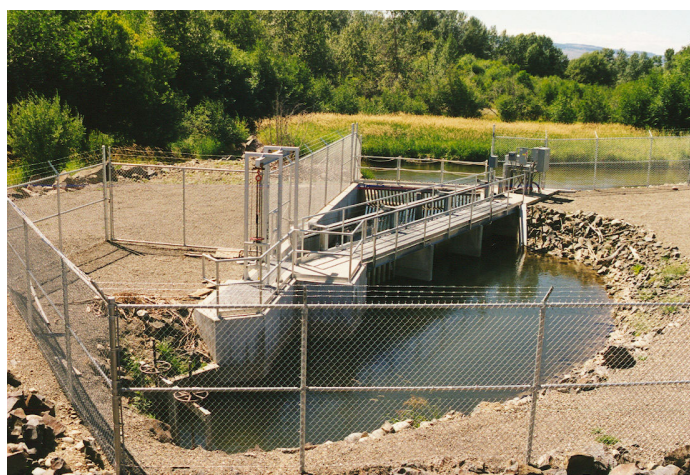
Figure 5.82: Water intake structure for irrigation purposes (Washington, USA): The water is led through a coarse screen to an inclined screen made of perforated plates ( d = 3.0 mm). The bypass is arranged at a pointed angle, and the fish are guided back into the water body through a pipe. The irrigation channel starts behind the sliding panel (on the left hand side of the picture)
