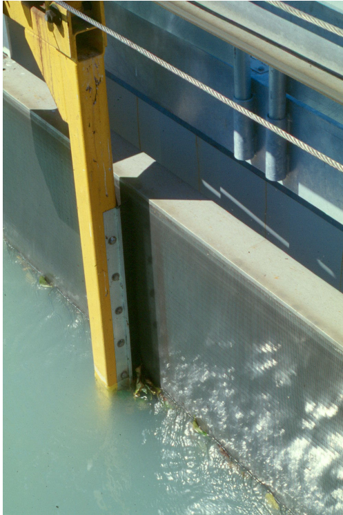
Figure 5.84: A Wedge-Wire-screen with a clear width of 1.25 mm and a brush-system at a facility with a design flow of 15 m 3 /s. The flow pattern illustrates the velocity component ( V_T = 0.34 m/s, V_N = 0.12 m/s) that acts tangentially to the screen. Hook river (Washington State, USA)
