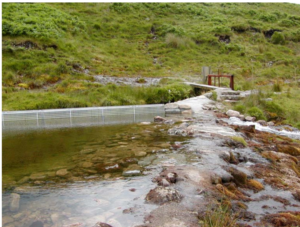
Plate 3.2 Fixed panel screen installed on the R. Plym, Devon in 2003, protecting the entrance to an industrial supply offtake.
