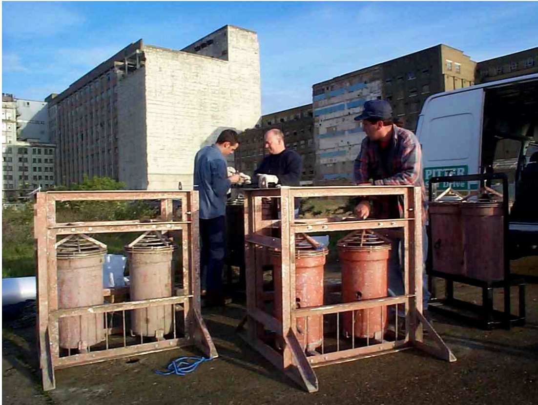
Plate 3.13 Acoustic sound projectors being prepared for installation at Amer Power Station (The Netherlands) (courtesy Fish Guidance Systems Ltd)
