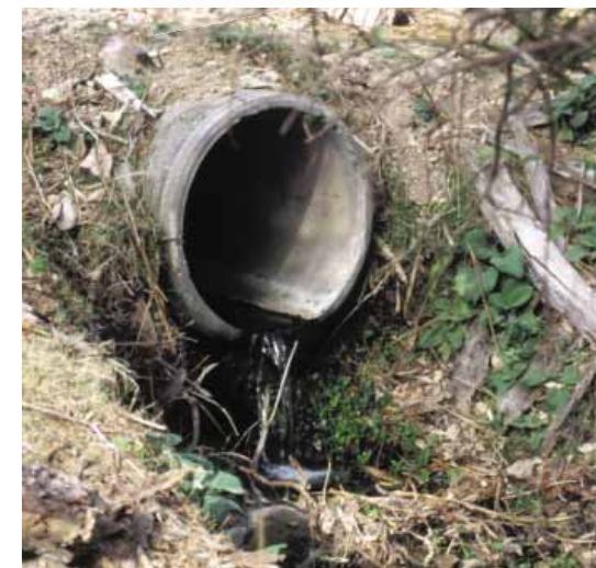
Fish can't migrate up a "perched" culvert
