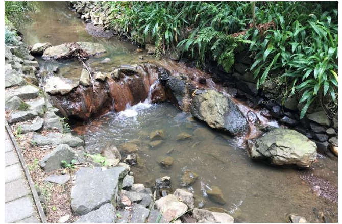
Figure 2: After installation of a concrete rock ramp to provide passage for swimming fish species, March 2016. Photo: NIWA
