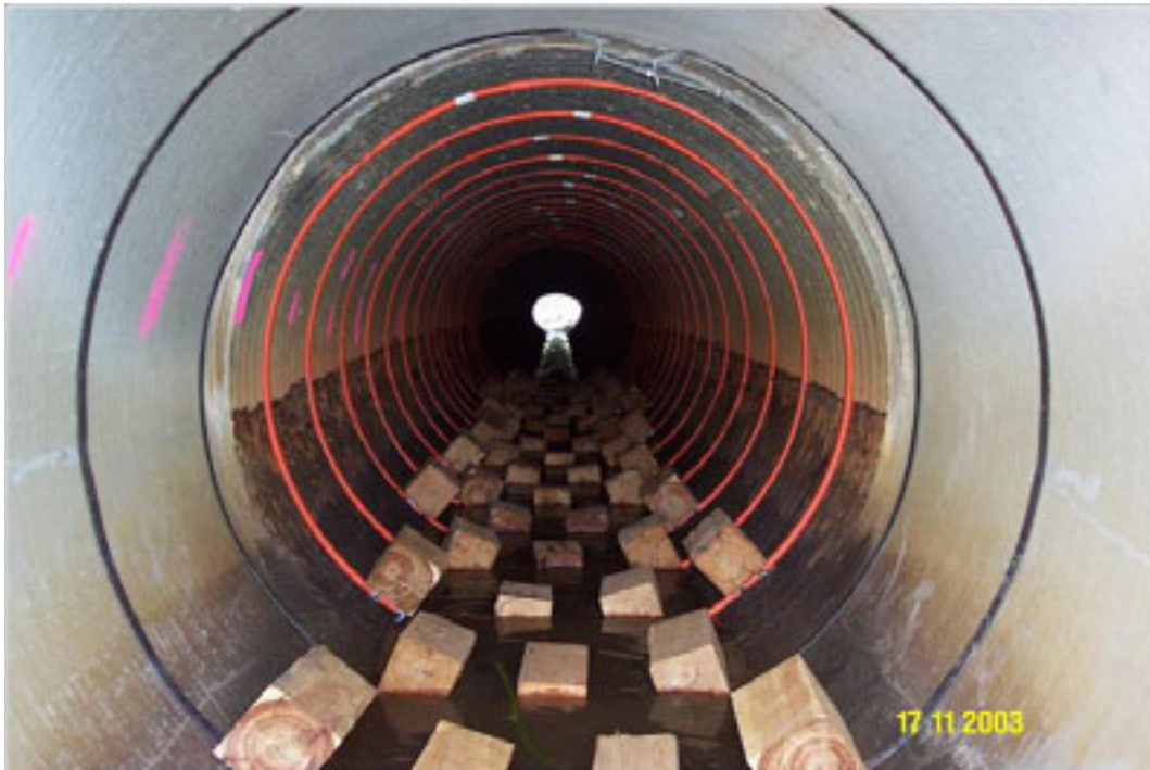
Figure 10 Baffles (these can be of many materials) and rocks can be installed into the base of a waterway crossing to provide cover and low velocity zones to aid with fish passage
