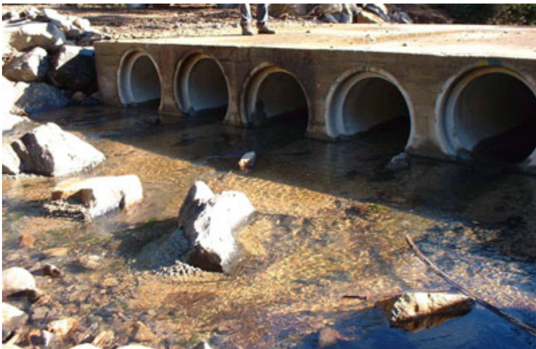
Figure 8 Multi-barrel circular culvert with culvert pipes at different levels to cater for high flows
