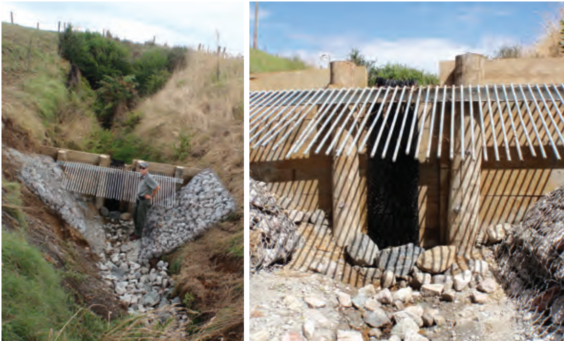
PLATE 4.8 Invasive fish barrier on Rotopiko (Serpentine) lakes outlet drain immediately following construction in early 2012. Left photo shows slotted timber construction, Reno mattress and grill bars. Right photo shows the upstream close-up view of the barrier.
