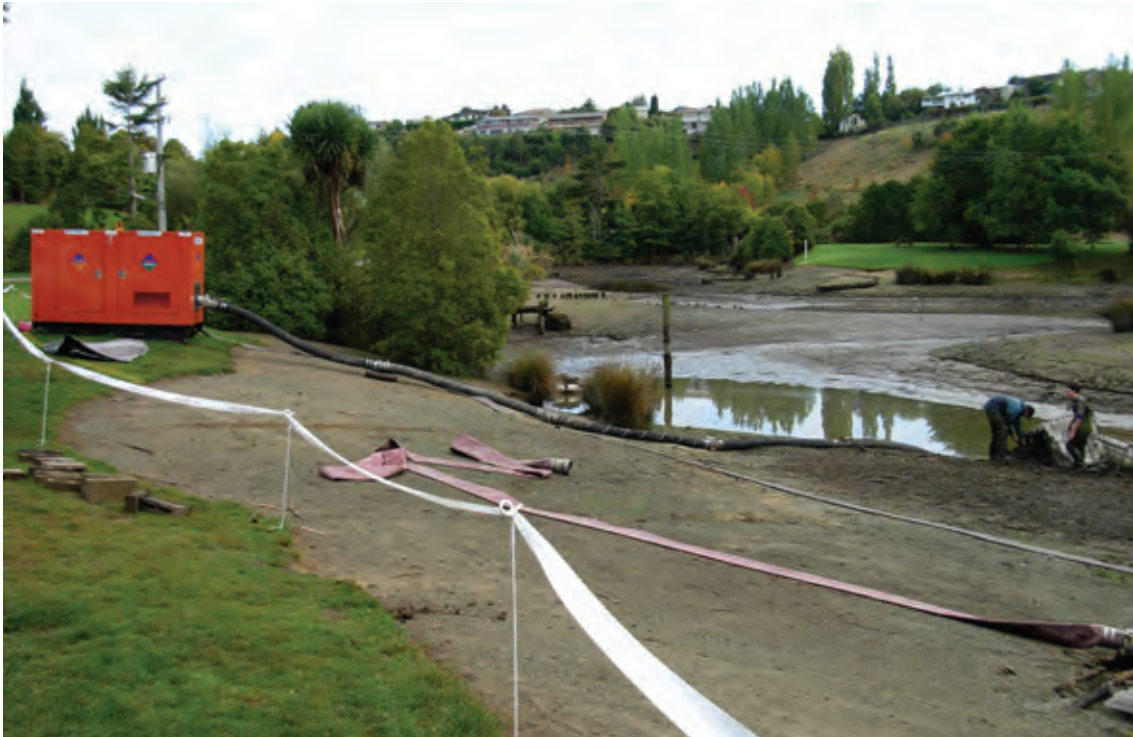
PLATE 4.3 Large industrial pump used to drain Centennial Park ponds, Timaru. Note: in this case the residual ponds were then treated with rotenone.
