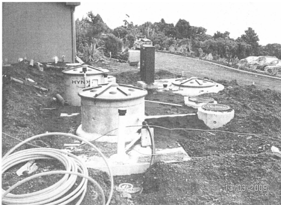
Figure 9: Hynds SAF wastewater treatment system installed in front of existing visitor centre (photo taken prior to backfill, from 2009 building consent)
