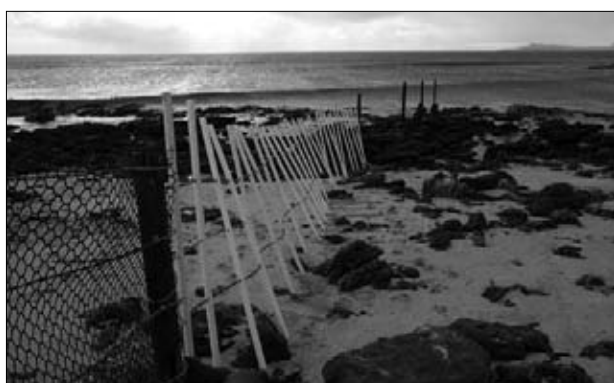
Figure 14. A fence tie-off extension of plastic poles designed to prevent stock entering Tioriori. Part of the original version of steel waratahs, wire cables and plastic mesh is visible to the left of the photograph, and concreted onto tidal rocks in the background. Photo: Peter Moore.
