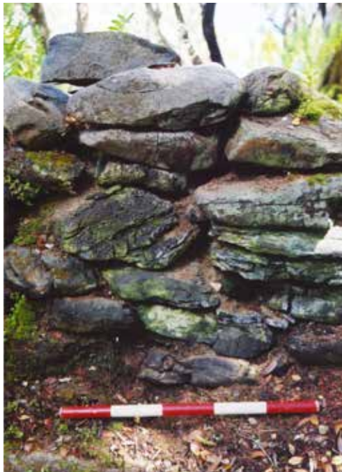
Figure 16. Detail of the in situ stonework of Epigwaitt hut in 2002. The lime mortar manufactured by Raynal in 1864 is still in place between these stones. Scale = 0.5 m. Photo: Peter Petchey.
