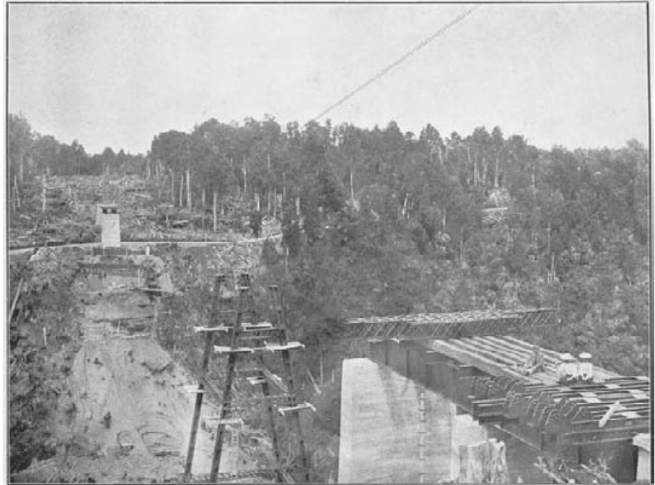
The main trunk line between Wellington and Auckland was officially opened by Prime Minister Joseph Ward on 6 November 1908. It was bounded by several scenic reserves as well as much land that is now part of the conservation estate. AJHR: Weekly Press, AJHR 1907, C6, opp. p. 9;
